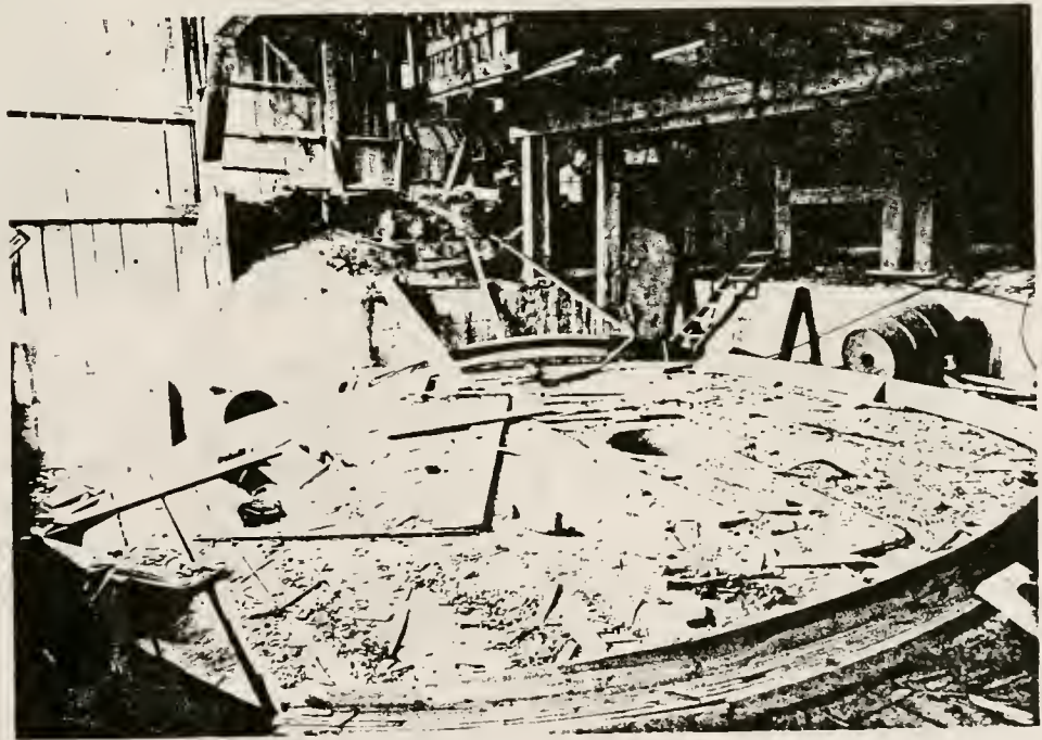
Figure 105. Revenue Mill (structure #34) interior - below flotation level - showing foundation rim of probable cyanide tank.
